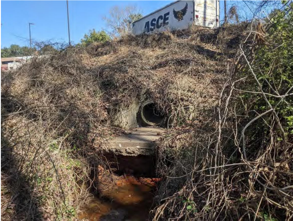
Photo 11: View of SW-M09 located off northwest corner of lot P23 near the Civil and Environmental Engineering building.
