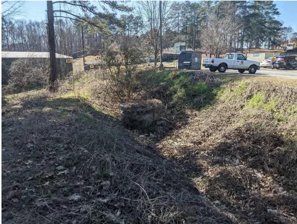
Photo 16: View of detention pond and outlet control structure (OCS19) discharging to SW-M13.
