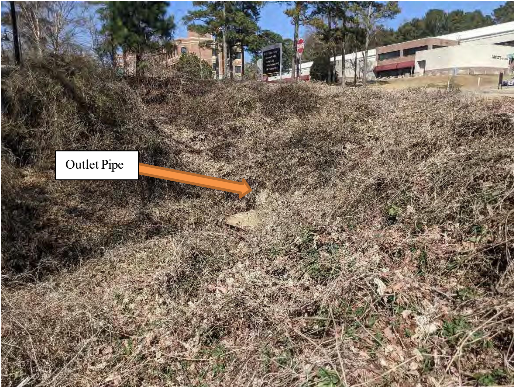
Photo 14: View of SW-M12 (outlet pipe) at the corner of Arnston Drive and Polytechnic Lane (entrance drive to Civil and Environmental Engineering building).
