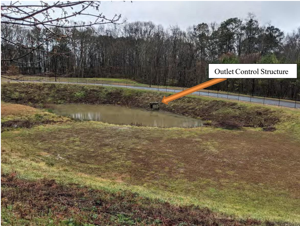
Photo 10: View of large stormwater pond and outlet control structure (OCS2539) near Hornet Village that discharges to SW-M08.
