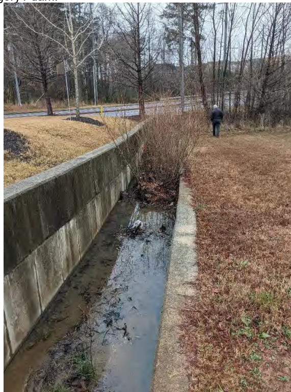
Photo 18: View of concrete channel located on southern portion of Nelson Pond emergency spillway.
