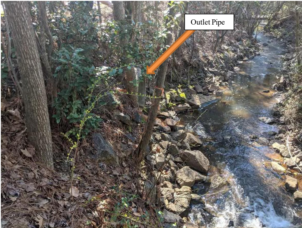
Photo 2: View of SW-K02 west of the Austin Residence Lot handicap parking area.
