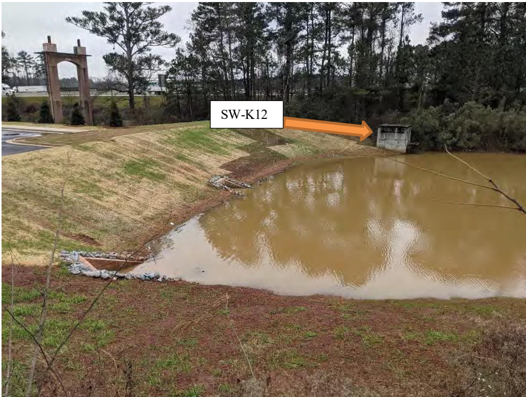
Photo 14: View of SW-K12 (outlet control structure) and southern portion of stormwater pond located near the Surplus building/ Shuttle Lot.
