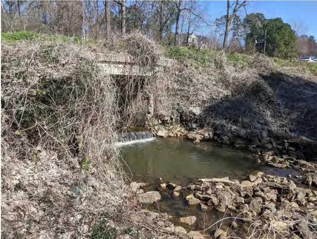
Photo 1: View of SW-K01 located behind Bowen Building, discharging under Campus Loop Road.
