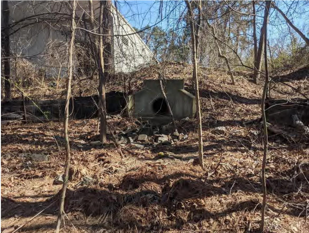
Photo 13: View of SW-M11 located on the southwest corner of the Student Competition Team building.
