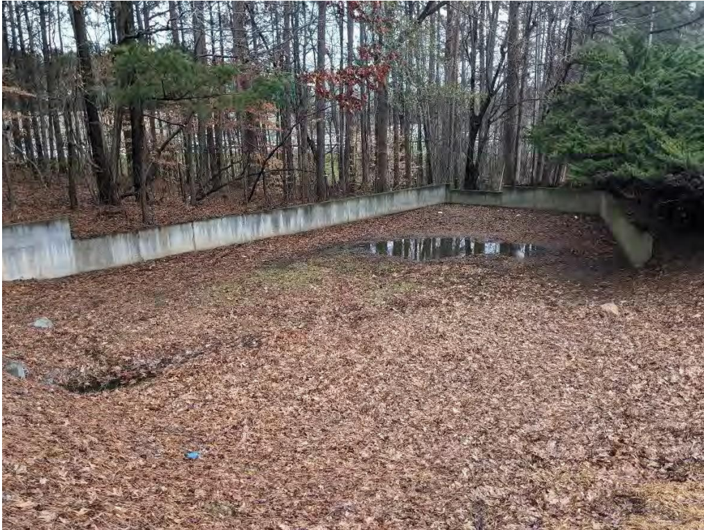
Photo 9: View detention area and outfall SW-K07 located south of KSU Place Apartments.
