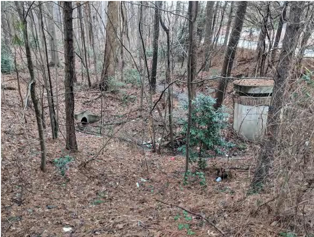
Photo 22: View of Outfall SW-K14 (outlet control structure) in detention pond located on southeast portion of Town Point.
